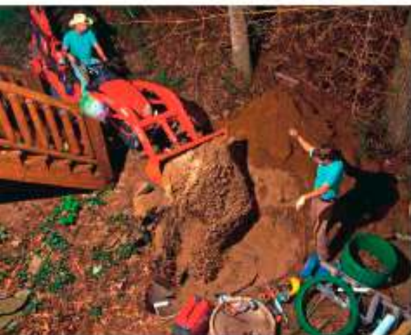
Heath Kilgore (left) and Justin Kilgore fill in with sand around a new Liberty Retro grinding station in Blue Ridge, Ga.
