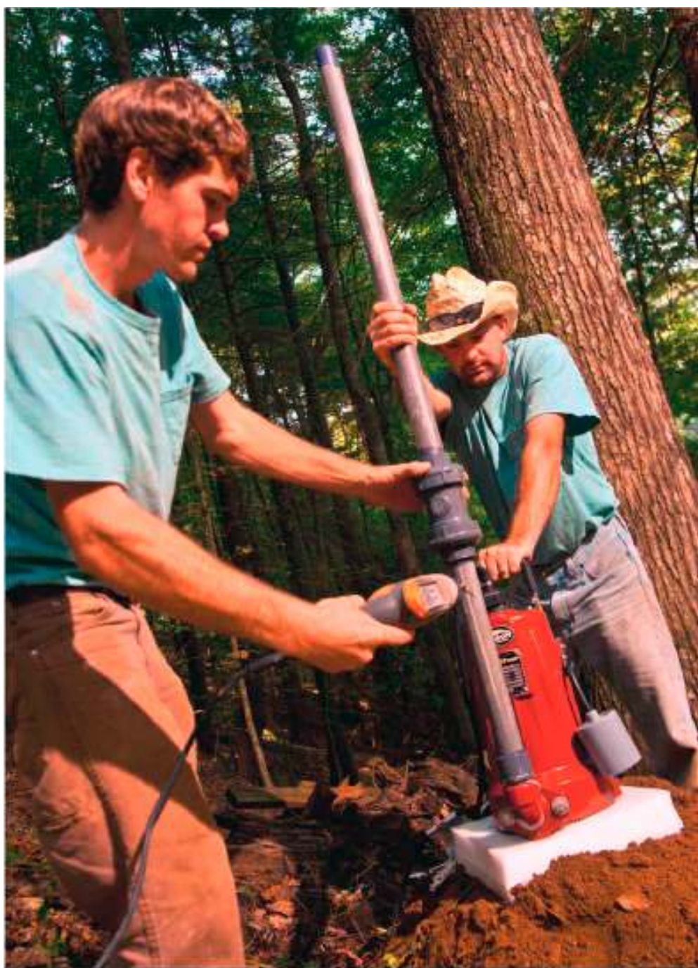
In the process of installing a Liberty pump in a new system, Justin Kilgore drills air release holes, while Heath Kilgore steadies the pump.
